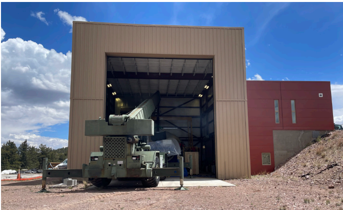
MROI team using a crane to help with the assembly of the dome and enclosure for the second telescope in the maintenance facility at Magdalena Ridge. The enclosure is being assembled by a team of engineers from EIE in Venice, Italy and will soon be integrated with the telescope and moved to the array arms.
