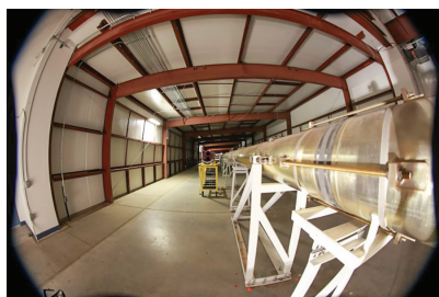
MROI Delay Line with the first 100 meter pipe installed in the Beam Combining Facility
